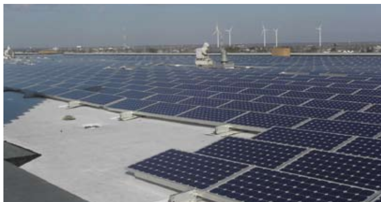
The Atlantic City Convention Center is one of the largest roof-mounted solar PV systems in North America, rated at 2.36MW of dc capacity. Higher valued SRECs enable profitable investments in solar without large rebates.
