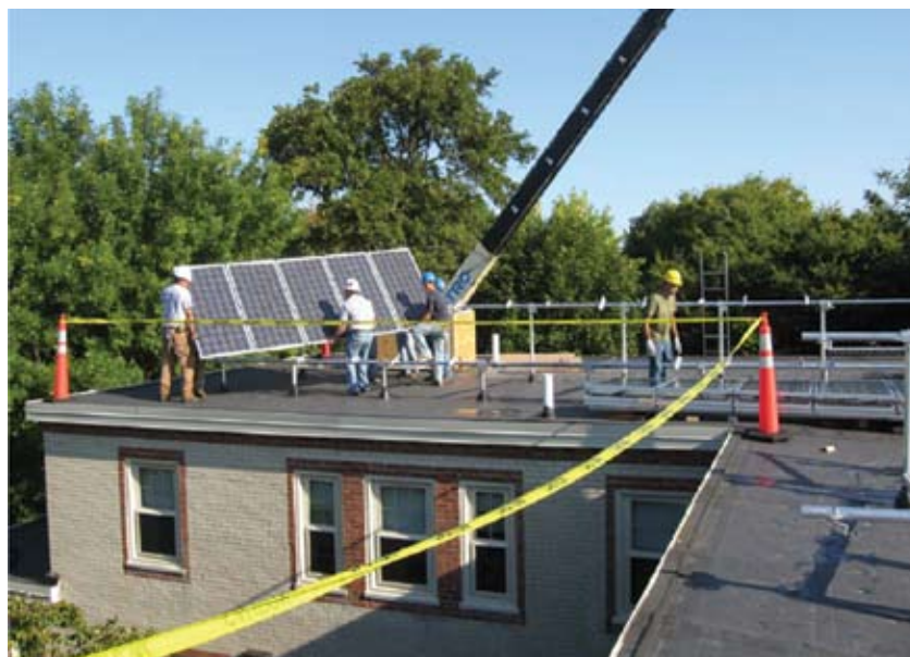
A 92-kilowatt solar system was installed at the Washington Elms affordable housing development in Cambridge. It will provide approximately 30% of the 145-unit facility's electricity.
