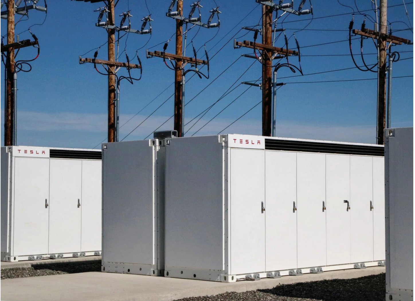
10.3 MW battery storage system owned by Brookfield Renewable located in East Millinocket, Maine, at the site of the former Great Northern Paper Mill. The nine Tesla Megapacks in this battery system have a capacity of 20 megawatt hours, about enough to power 9,000 homes for two hours.
