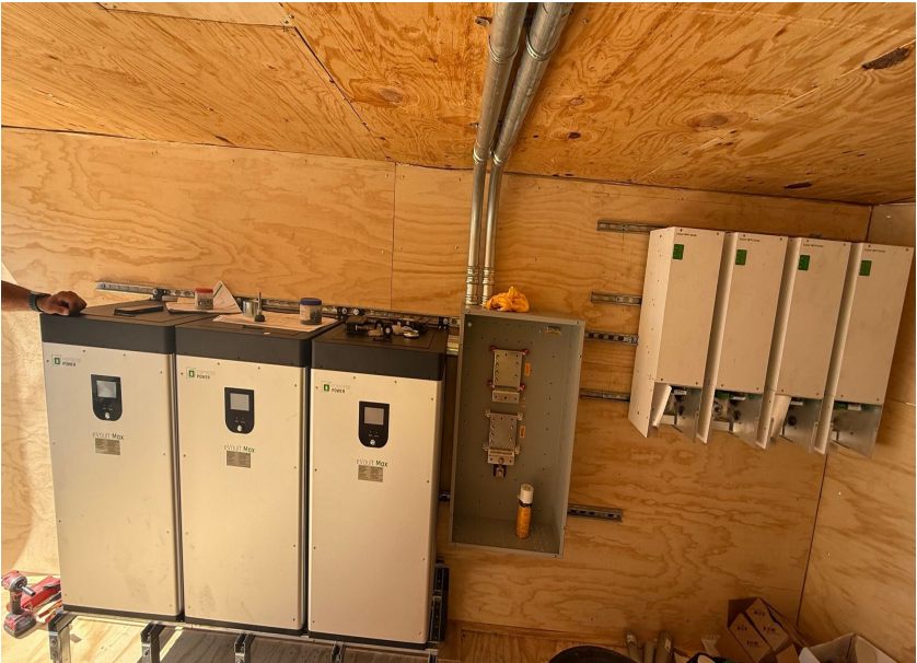
Fortress Power eVault Max battery bank (BESS) installed inside the trailer
