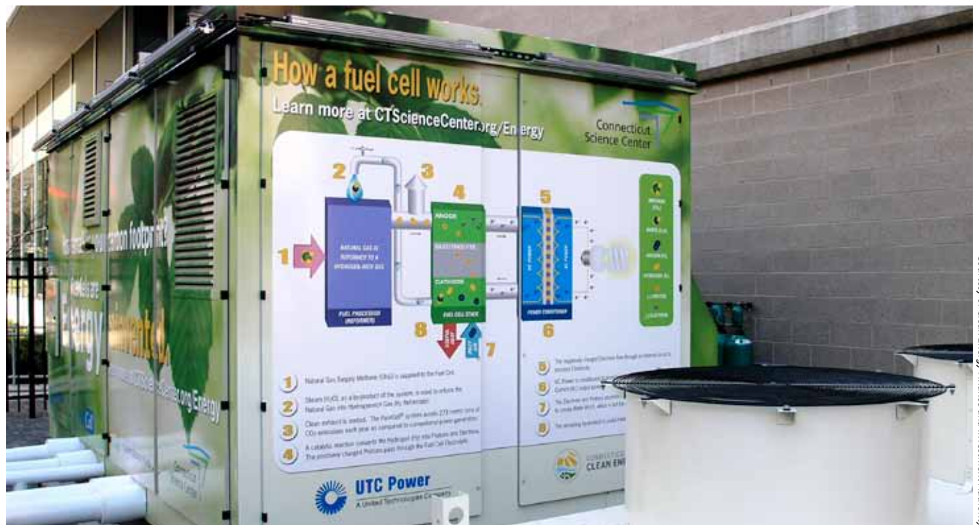
Connecticut Science Center, Hartford. This 200-kilowatt fuel cell at the new Connecticut Science Center will generate almost 100% of the electricity used at the science center annually.
