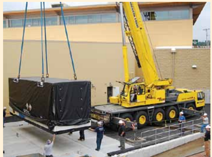
A fuel cell being delivered and installed at the Whole Foods Market in Dedham, Massachusetts.
