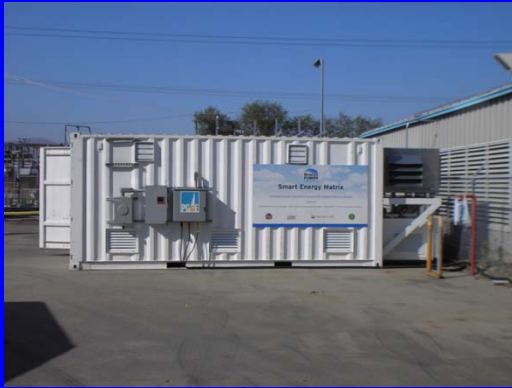
CEC/DOE: 100kW Beacon Flywheel Demo
