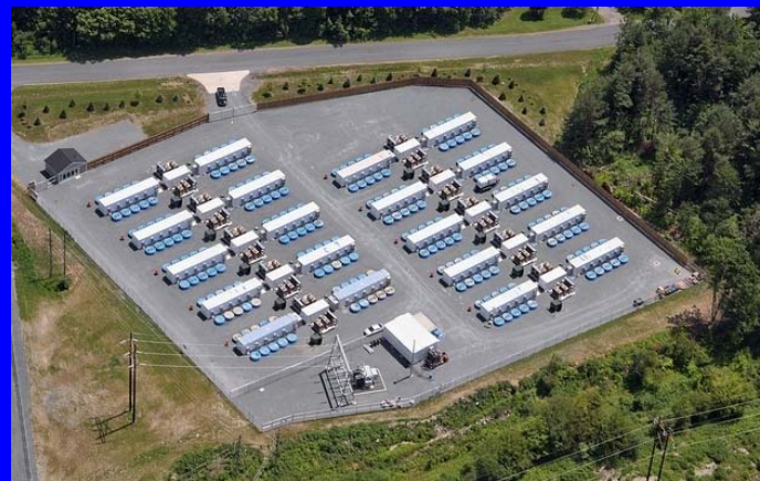
DOE ARRA: 20MW Beacon Installation
