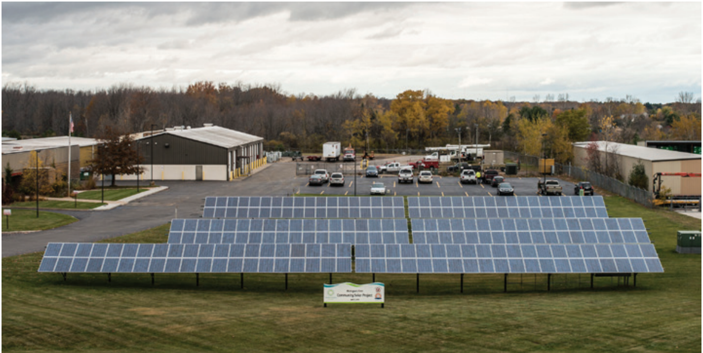
Cherryland Electric Cooperative's Grawn community solar array. Photo: Cherryland Electric Cooperative
