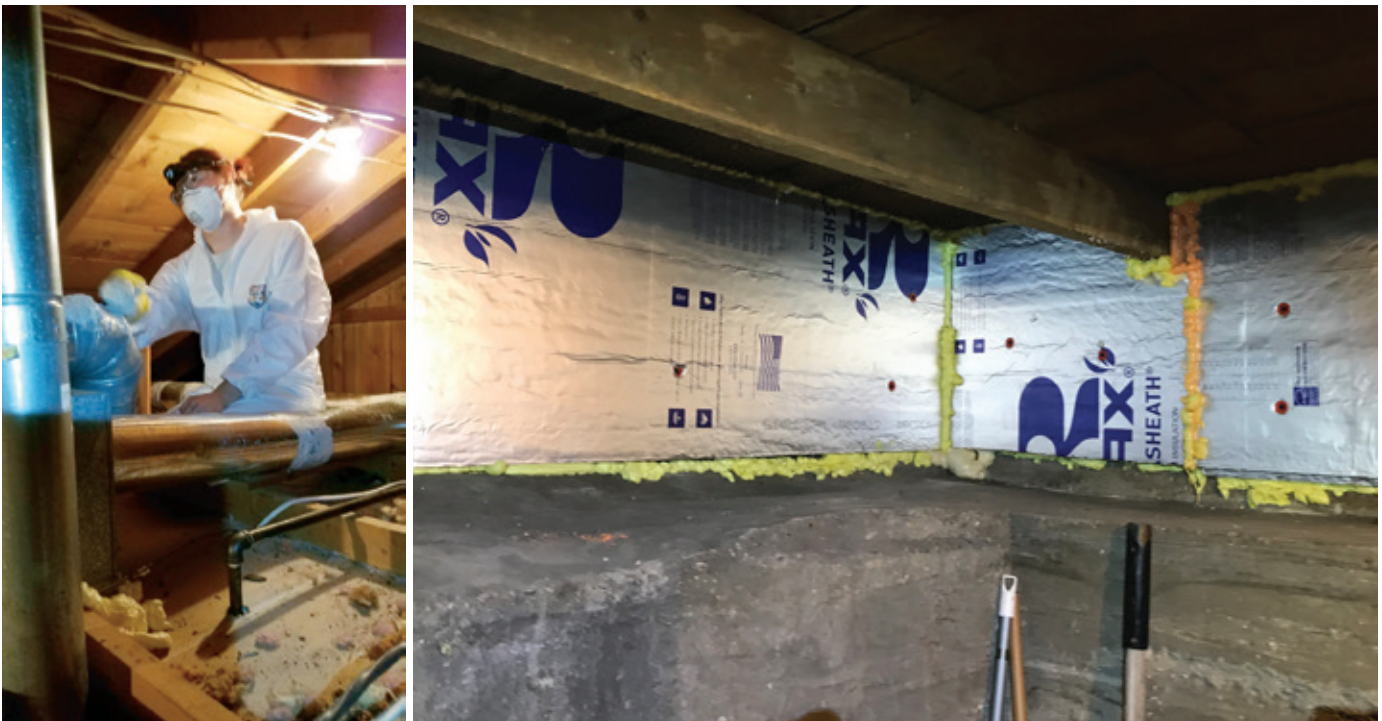
Left: Weatherization crew member performs air duct sealing in home being Weatherized. Sealing and insulating leaky air ducts increases energy efficiency and can lower monthly utility bills. Right: Foundation insulation after a home has been Weatherized: foil-faced insulated boards, air-sealed around the edges, prevent cold from entering the basement in this home. Photos: Northwest Michigan Community Action Agency
