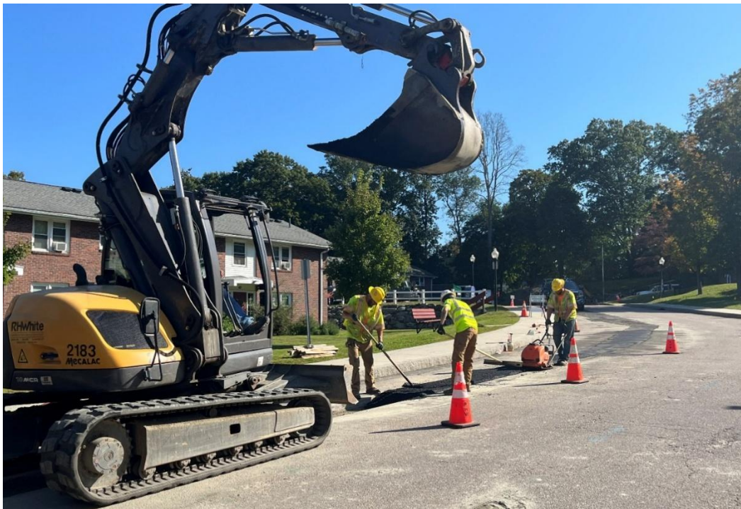
A geothermal pipeline is installed beneath a road in Framingham, MA. Credit: Eversource Energy.
