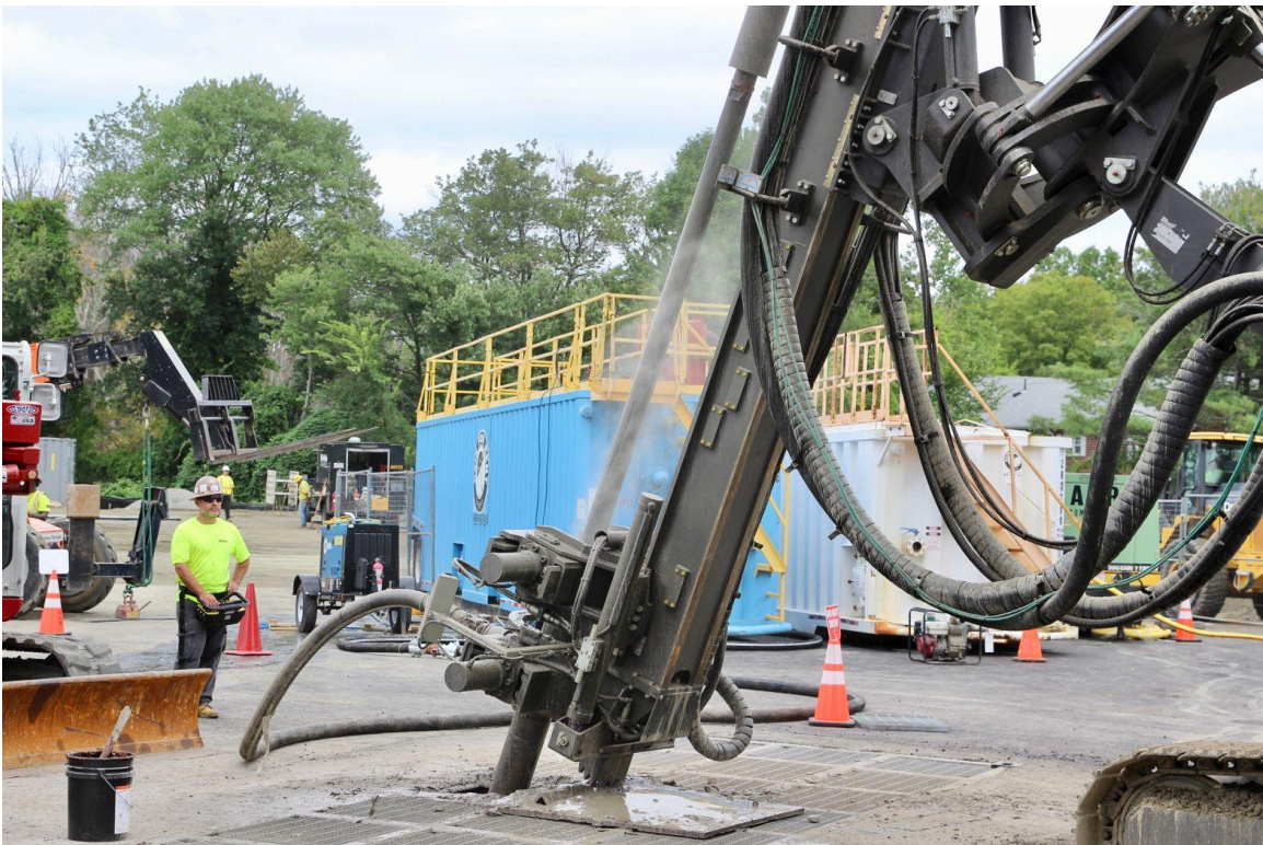
Borehole drilling for a networked geothermal project in Framingham, MA. Credit: Eversource Energy.
