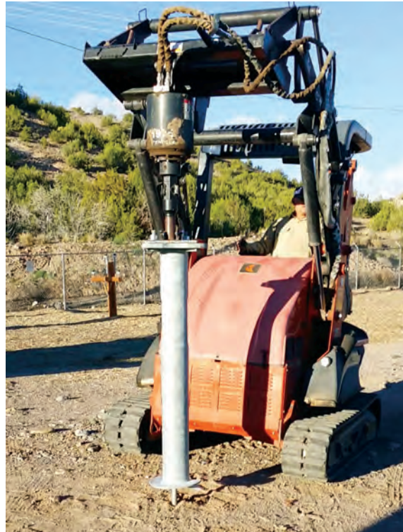
Light pole foundation attached to the driving machine, ready to install. Machine and operator courtesy Jemez Mountain Electric Coop.
