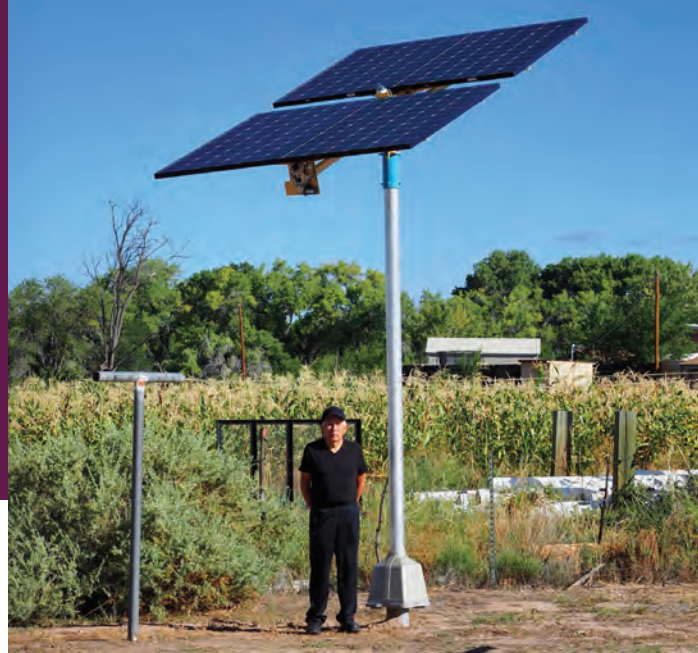
Victor Perez stands next to his PV on a Pole installation at Nambe Pueblo, New Mexico.
