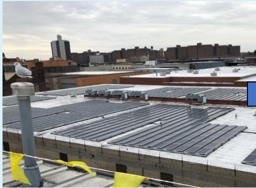
Community Solar System
